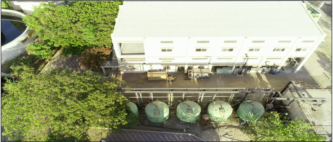
This PSF filters and RO
